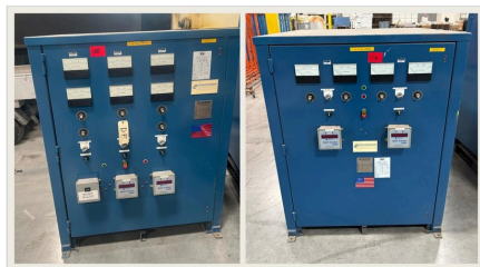
Dynapower water-cooled SCR rectifiers. Three-circuit and two-circuit cabinets.
