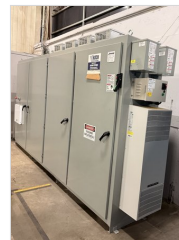
Control cabinets, new in 2024.
